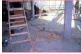
Cables or hoses left on floors
