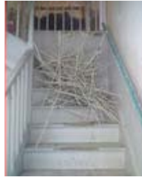
Debris piled on stairs
